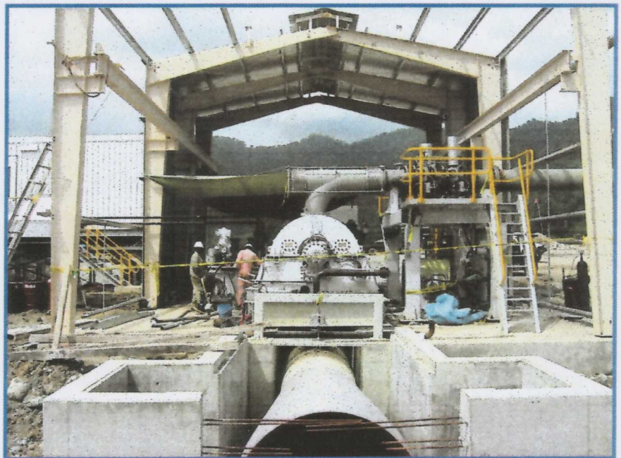
Powerhouse under construction showing the turbine and pressure balanced inlet elbow, and inlet steam valve maintenance platform. The atmospheric exhaust duct can be seen in the lower foreground.
